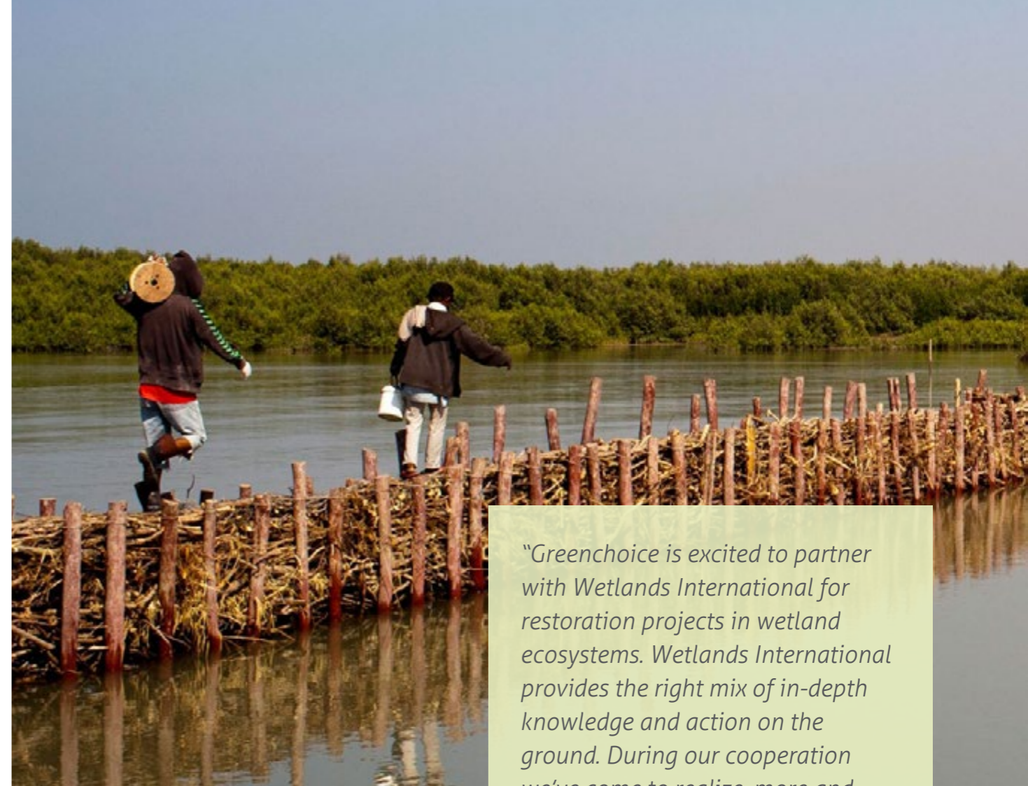
Villagers assist in building and maintaining brushwood barriers along the coast of Java, with assistance from Wetlands International. Such actions reduce the risk of future flooding in the region.
