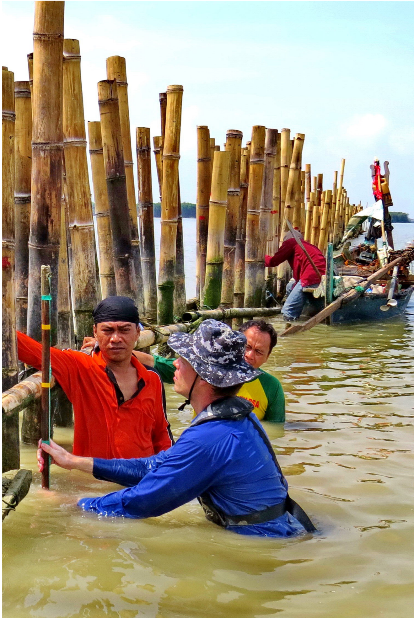
Community establishes permeable structure to catch sediment to let mangroves grow back naturally.
